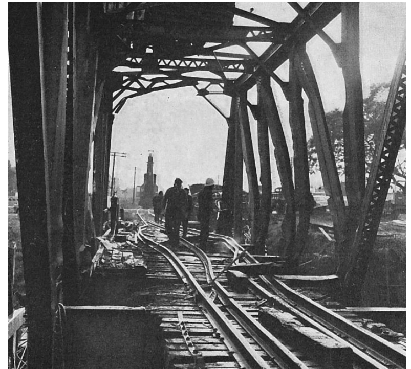
Figure 3 – Guard rails failed to protect through truss span 11
