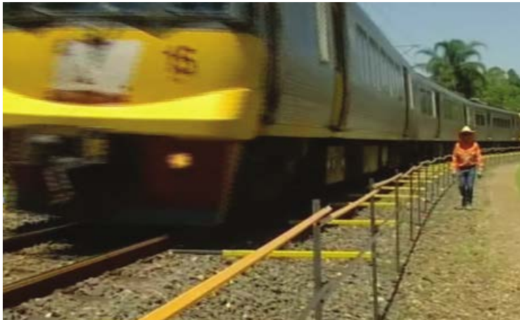
Figure 1 - The use of SAFETRAX Temporary Handrail System as a demarcation fence is a means to reduce risk and aid in the protection of workers from rail traffic.
