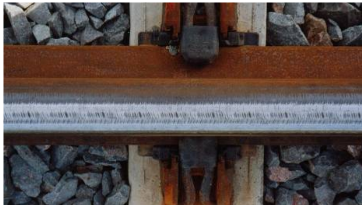
Figure 13: Example of Unacceptable Cyclic Grinding Scratches
