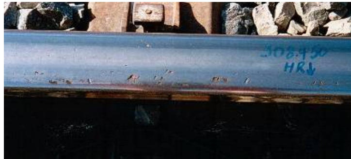
Figure 11(a): Example of Moderate Gauge Corner RCF Defects on High Rails Requiring Application of the ARTC H2 Profile
