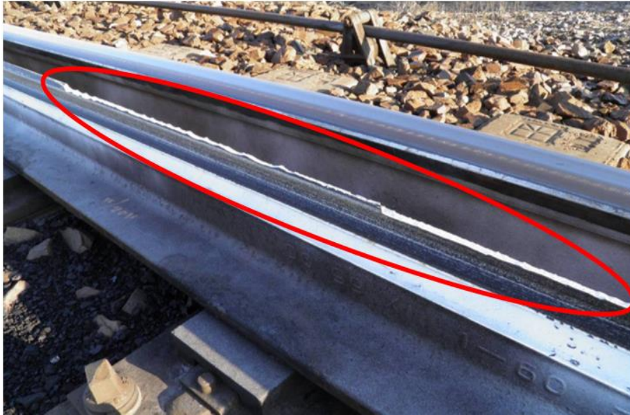
Figure 3-2: Switch blade with pieces broken away
