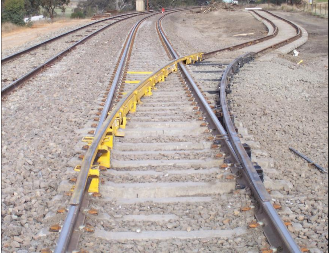
Figure 1 – Photo of Temporary Take Off Installed Ready for Use
