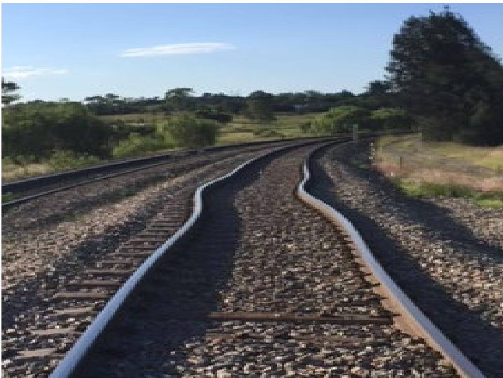
Figure C1 - Track clearly showing a buckle
