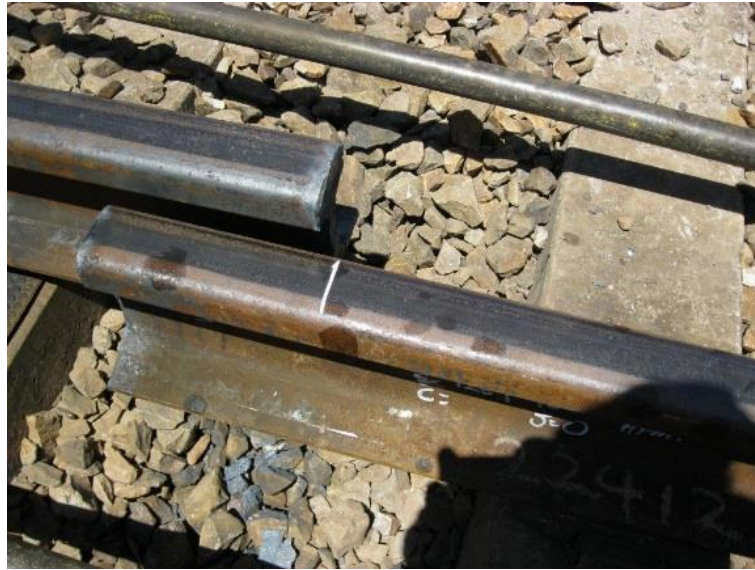
Figure 7 - Overlapped rail with contact only maintained at the web
