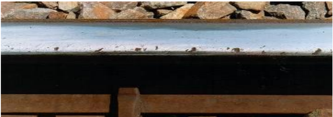
Figure 6 – Example of severe gauge corner RCF on high rails that may require application of the H3 profile
