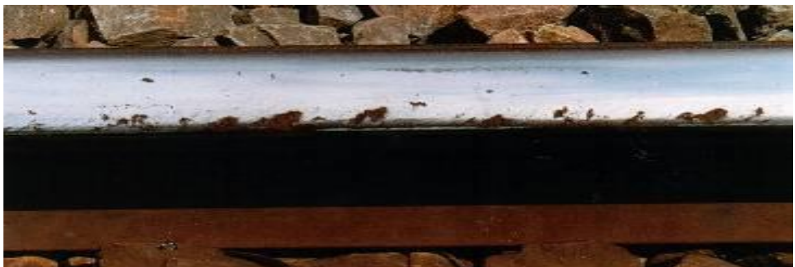
Figure 9 – Severe gauge corner RCF defects on high rails requiring application of the H3 profile
