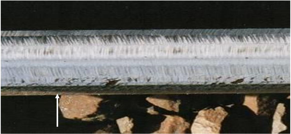
Figure 5 – Example of gauge corner checking defects left in the high rails after transitional profiling (arrow points to the gauge corner)
