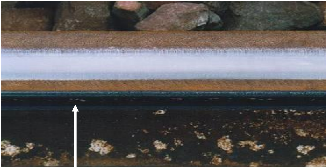
Figure 10 – Unacceptable gauge corner undercutting on high rail in sharp curve (arrow points to gauge corner)
