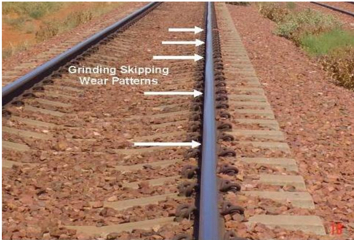
Figure 22 – Cyclic wear (skipping) induced by rail profiling
