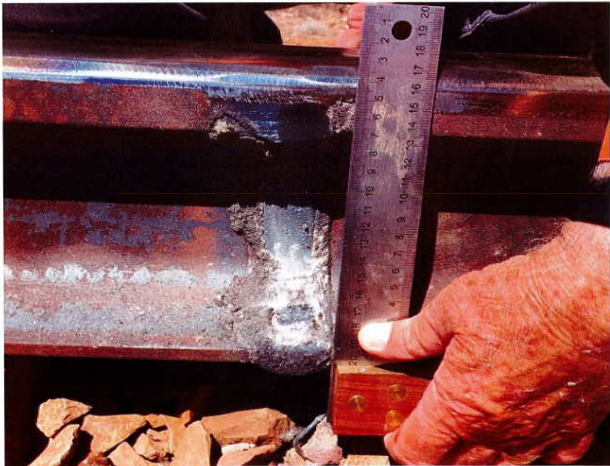
Figure 1: Poor vertical alignment
