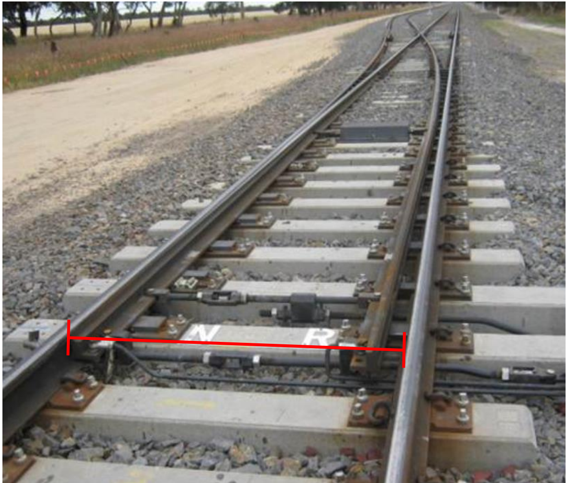
Figure 4-3 Track gauge at the switch tip
