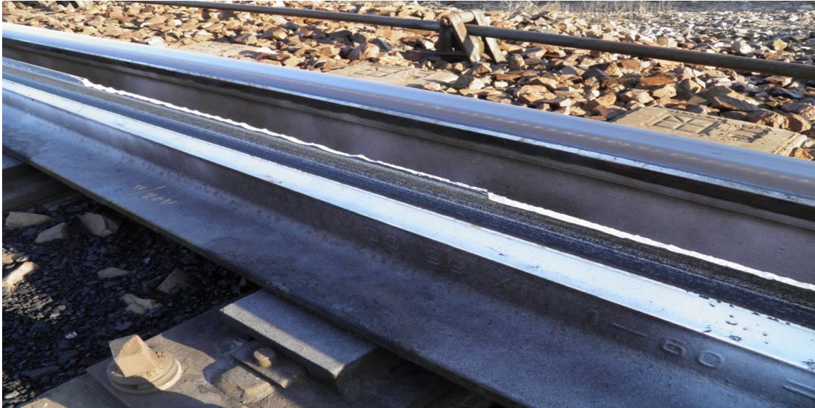
Figure 4-9 Switch Rail Head Damage Resulting from RCF Cracking
