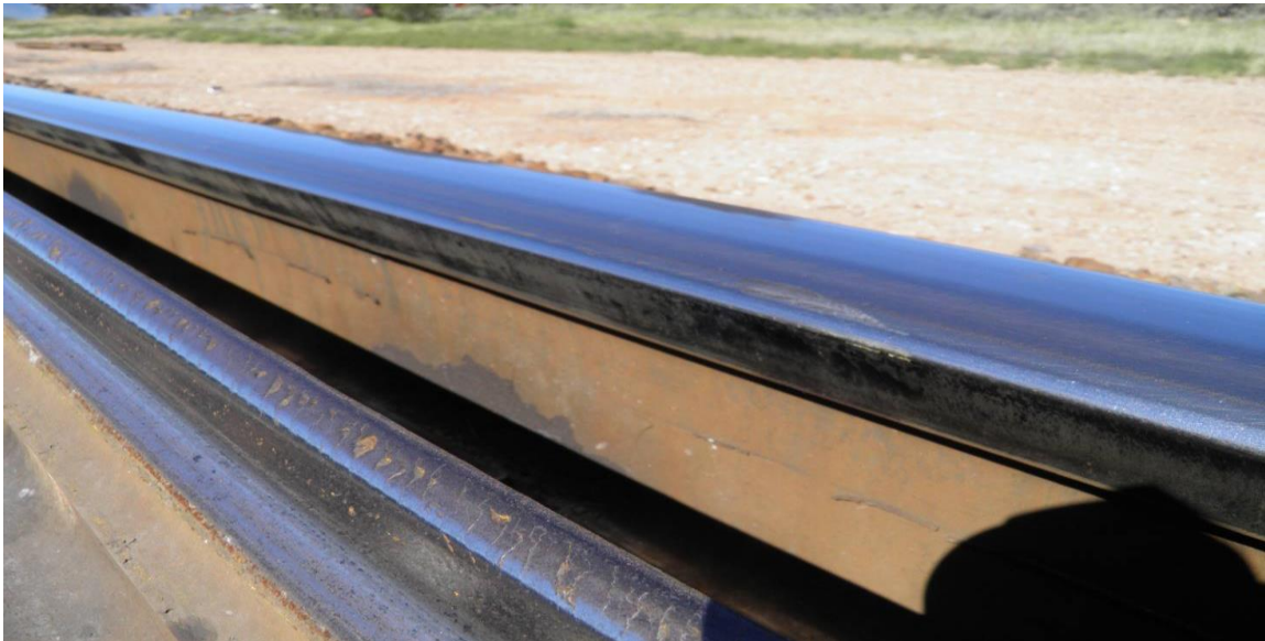
Figure 4-8 RCF Cracking on Head of Tangential Switch Blade
