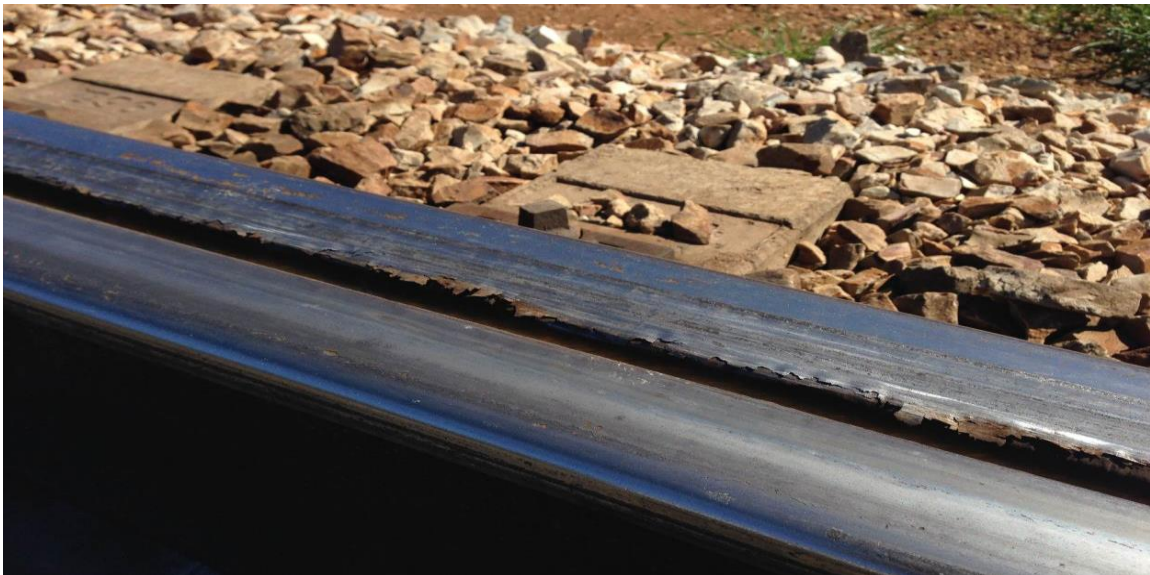
Figure 4-10 Damaged Stock Rail
