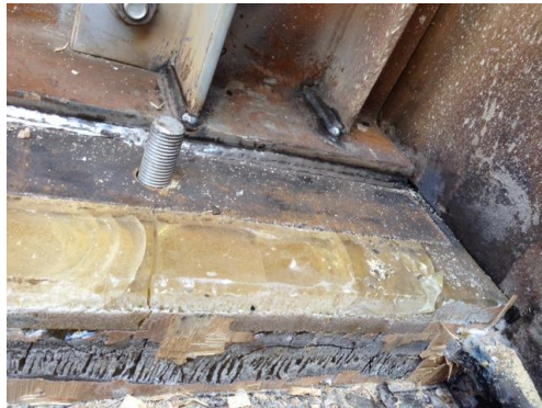
Poorly formed Bearing Pad - honeycombed
