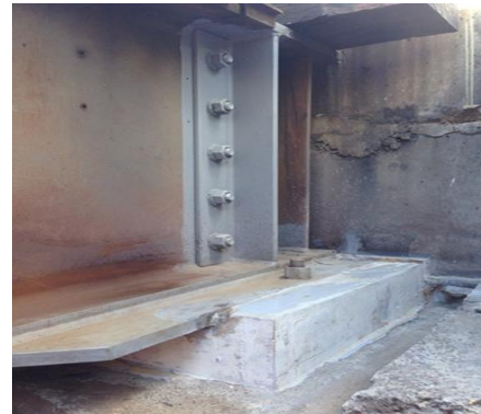
110mm thk Megapoxxy Bearing Pad with 75mm dowels confined by SL81 mesh
