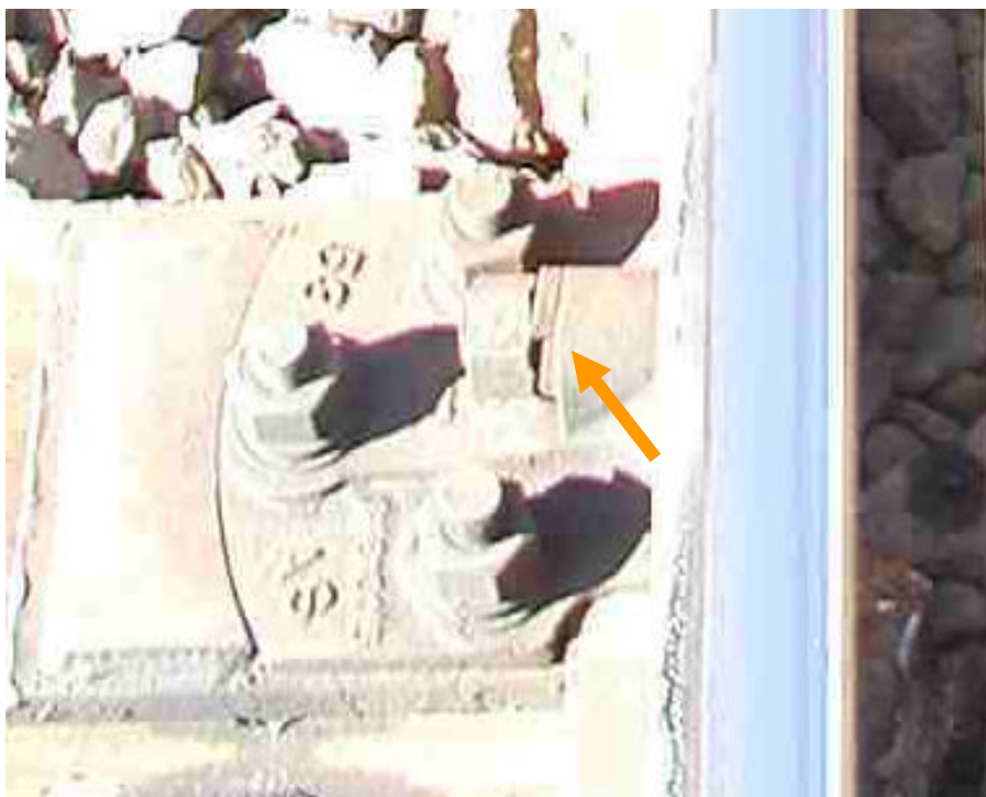
Figure 2 – Bolts Loose - washer not fully compressed
