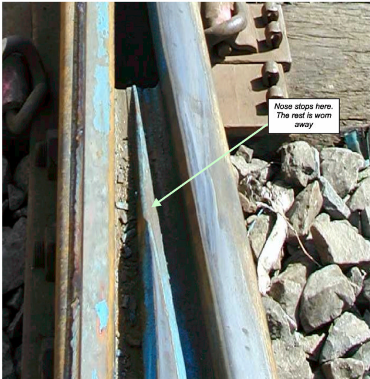
Figure 2. The ramp and nose of the K Crossing have been completely worn away. Note that the wingrail on the LHS has been raised to reestablish checking for the diamond.
