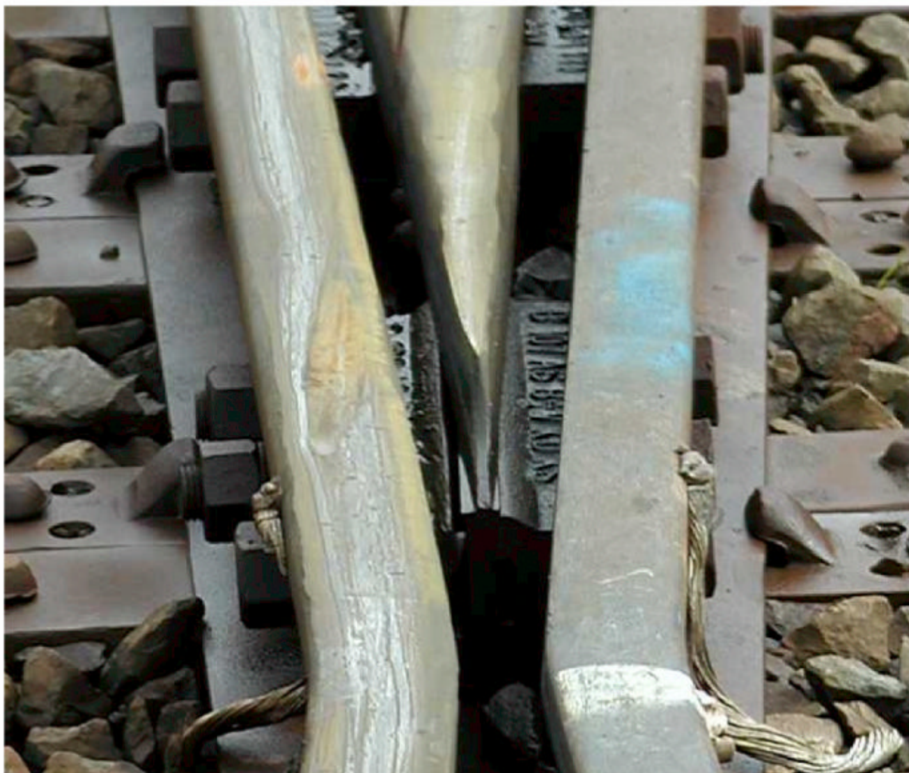
Figure 1 A typical K Crossing nose in Category 3. The ramp up to the nose is worn and rolled over.
