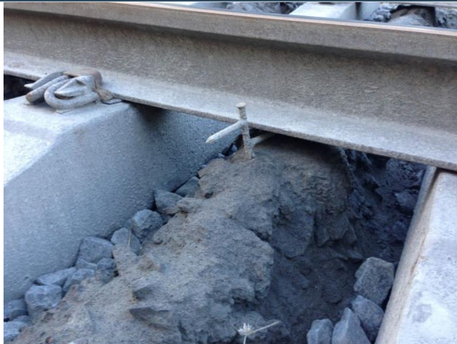
Figure 2: Type 2, Depression peg (simple assembly of a sharp spike), after passage of a train.
