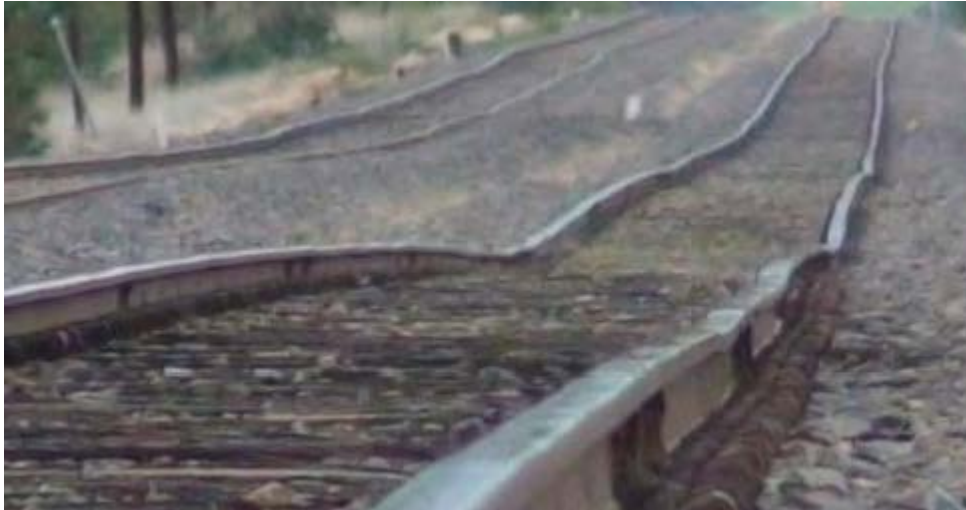
Photo 2.2.2 – Soft formation mud hole (refer to drainage manuals listed in clause 1.5)
