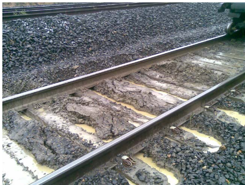
Photo 2.2.1 – Fouled ballast type mud hole (This is a perched type with water and mud in pockets around the sleepers)
