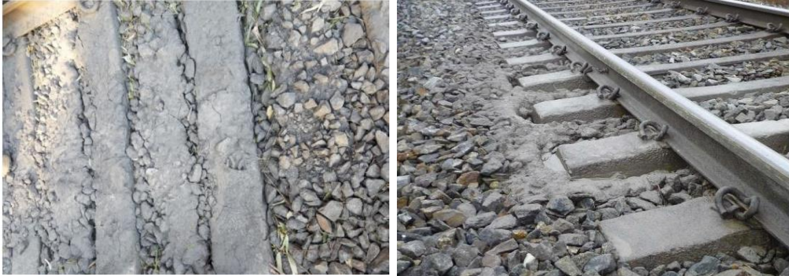
Figure 1: Sleepers covered with mud and visible gap present around the sleepers and evidence of pumping
