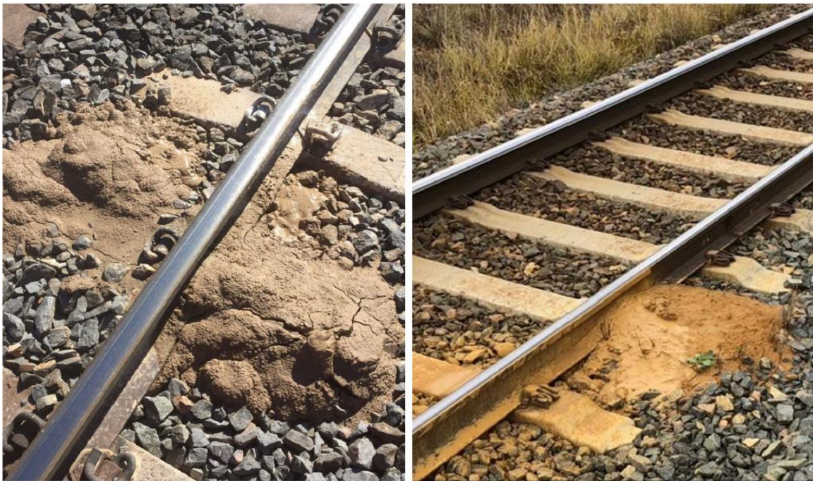
Figure 7: Brown mud accumulating on the surface of the ballast, signalling potential issues with the formation or capping layer, and early signs of drainage failure
