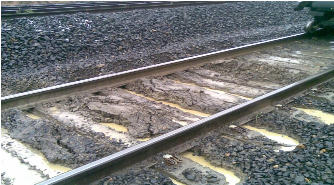
Figure 4:Fouled ballast mud hole (This is a perched type with water and mud in pockets around the sleepers)
