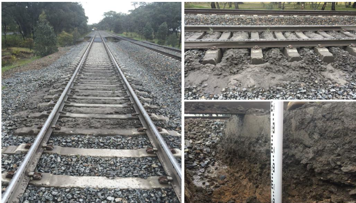
Figure 5: Sleepers enveloped in grey mud, a clear sign of ballast degradation
