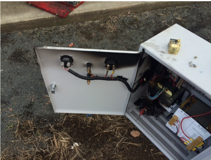
Figure 1: Capacitor failure and fire in Store 74 battery charger.
