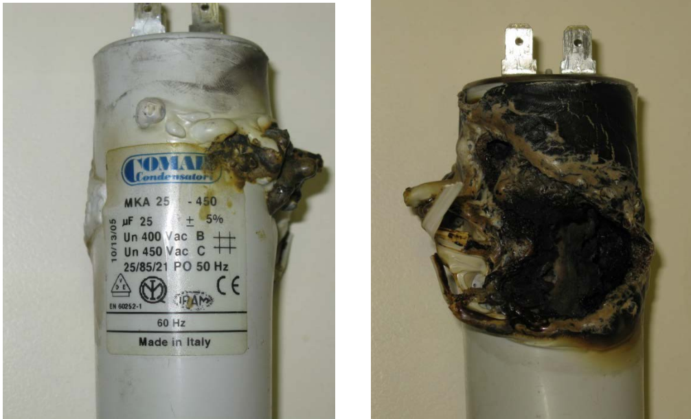
Figure 2: Failed resonating capacitor. Front and back.
