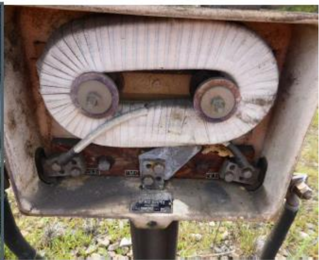
Figure 2: Internal view of UM71(CSEE) SI Unit
