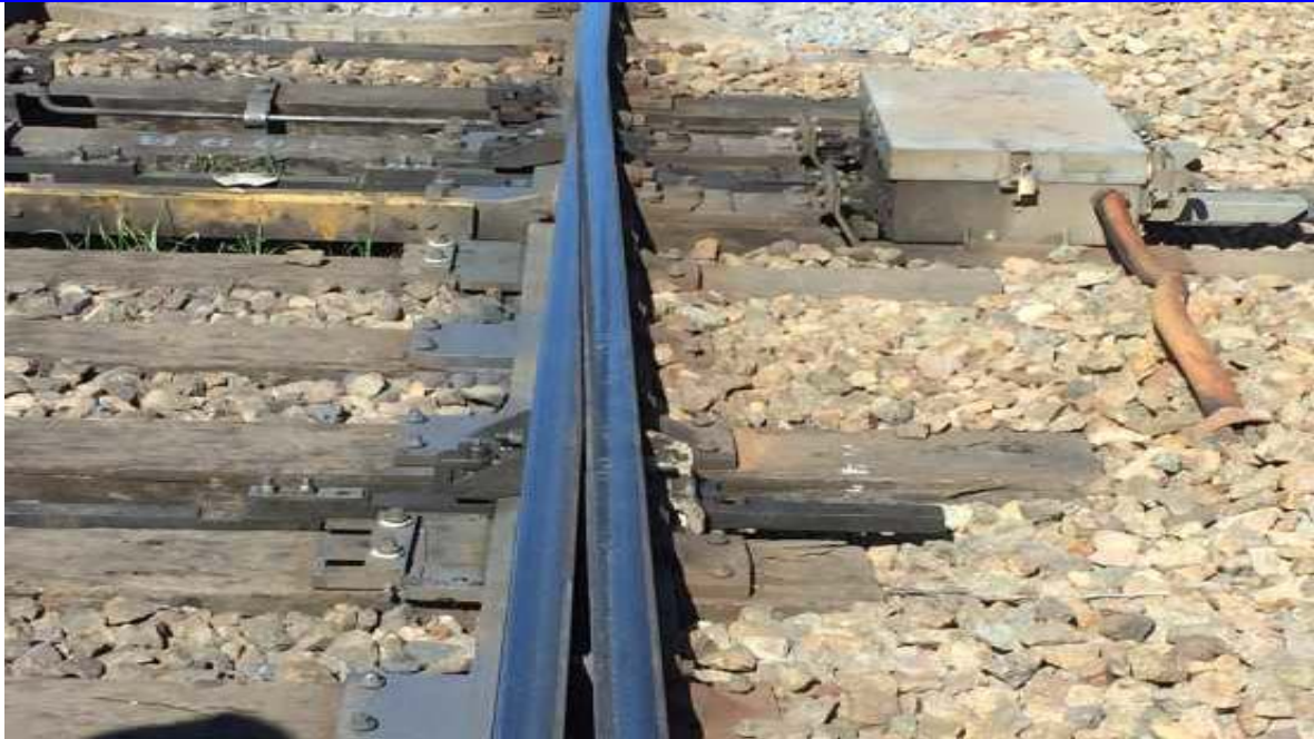
Fig 3. Incorrect coupling bar installed to turnout.
