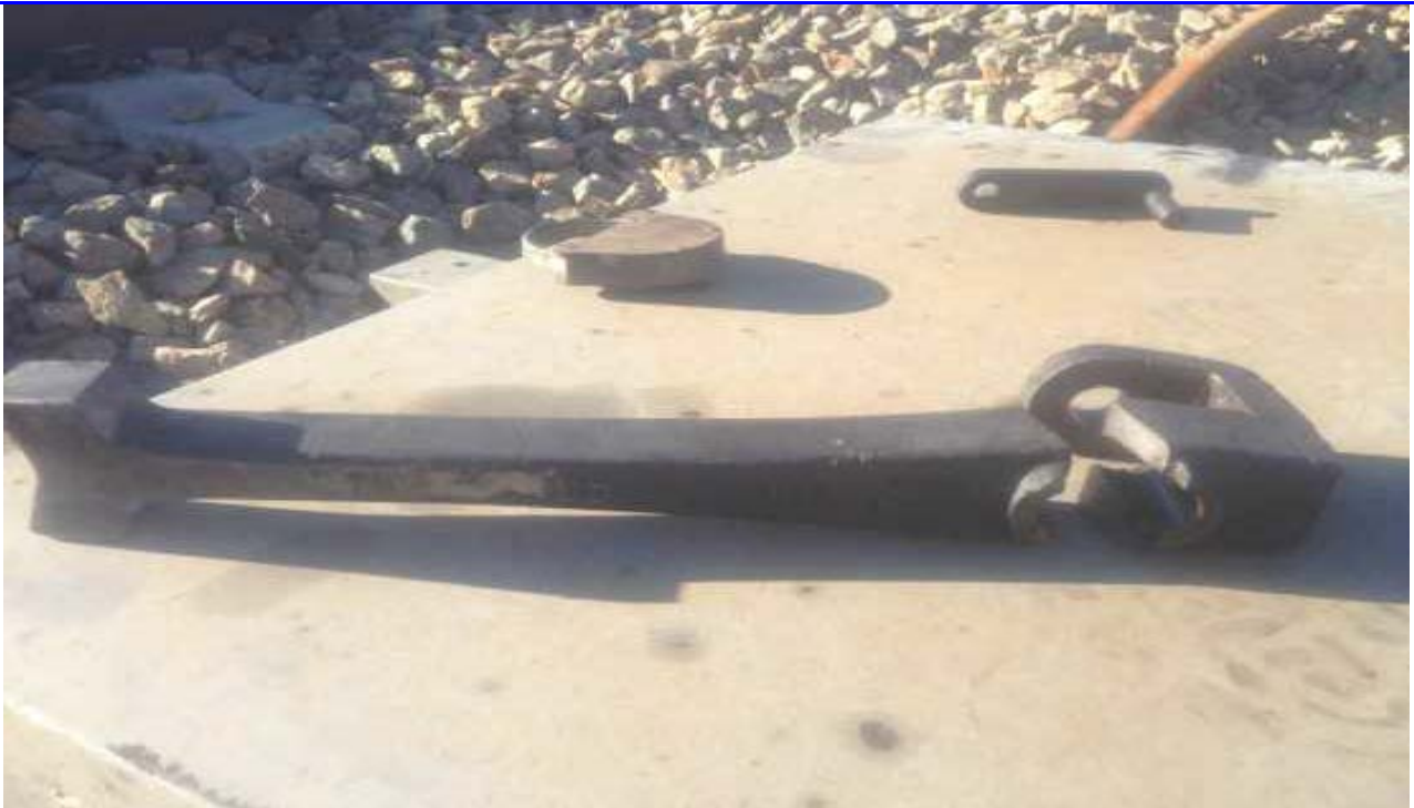
Fig 1. Points were pumping at the B and C timbers, which caused excessive stress and wear causing subsequent failure of the claw (See Above).
