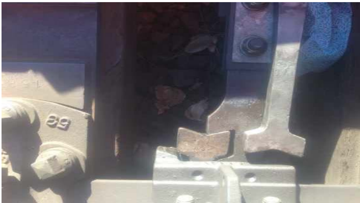
Fig 2. Claw has been ground to allow locking to occur due to incorrect lock box installation.
